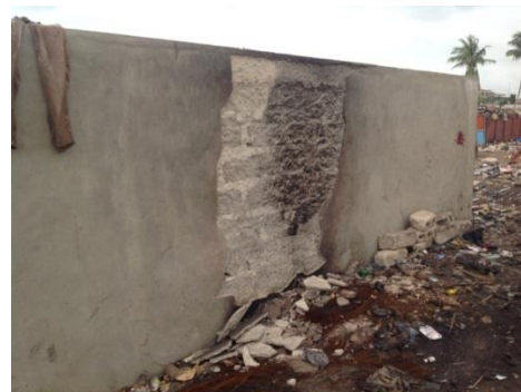
Photo 9 : Eroded wall and swish by waste incineration fumes in Sèdjèko
